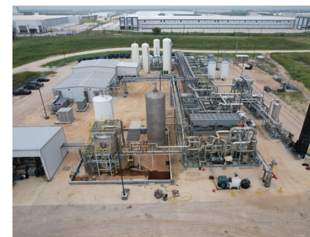
Tessman Road RNG 1.2M MMBtu Texas, USA
