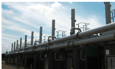
Pitsea Landfill Gas Power Station 12MW, Essex, UK
