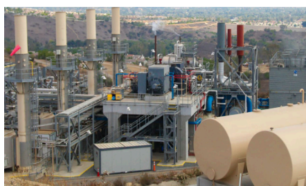
Brea Landfill Gas Plant 32MW, California, USA
