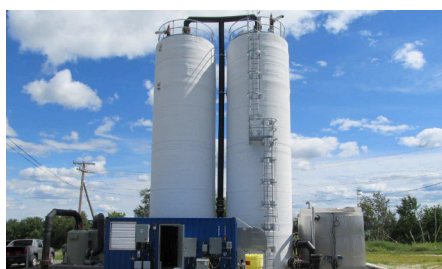
Lidya Landfill Gas Power Station 11MW, Quebec, CA
