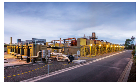
Lucas Heights Landfill Gas Power Station 17MW, New South Wales, AU
