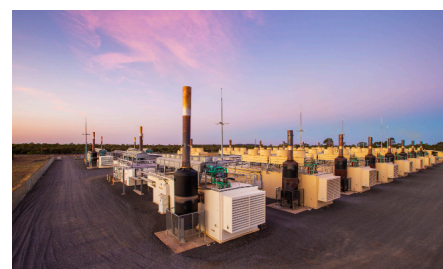
Moranbah Waste Coal Mine Gas Power Station 64MW, Queensland, AU
