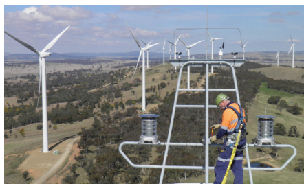
Cullerin Range Wind Farm 30MW, New South Wales, AU
