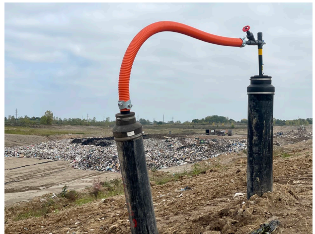
RNG will be created from waste gases from Granger Waste Services' Wood Street Landfill
