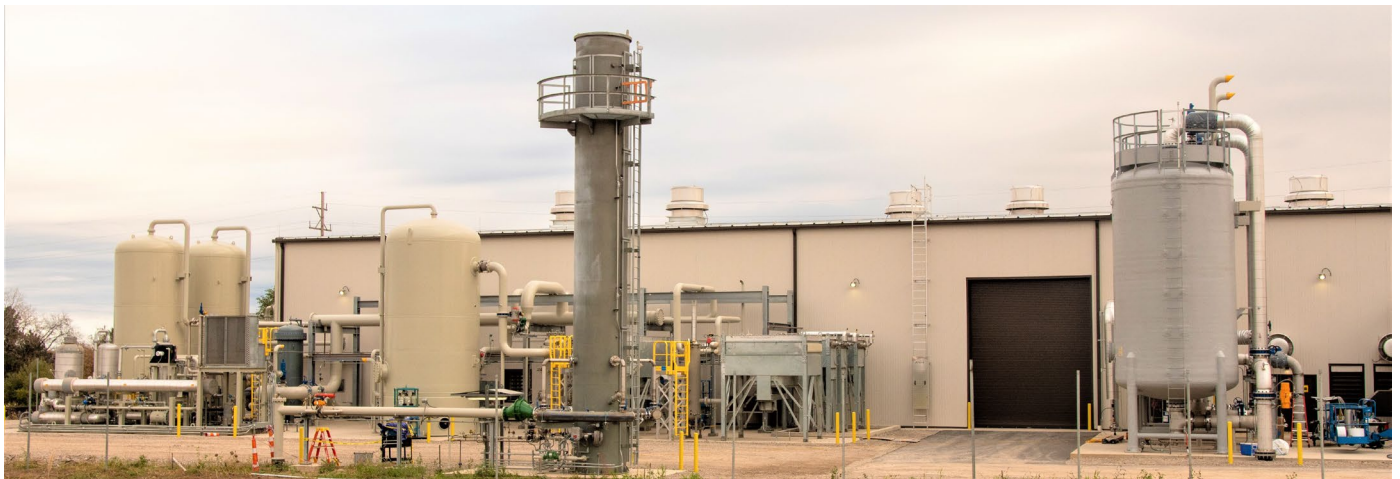
EDL's Wood Road RNG Facility
