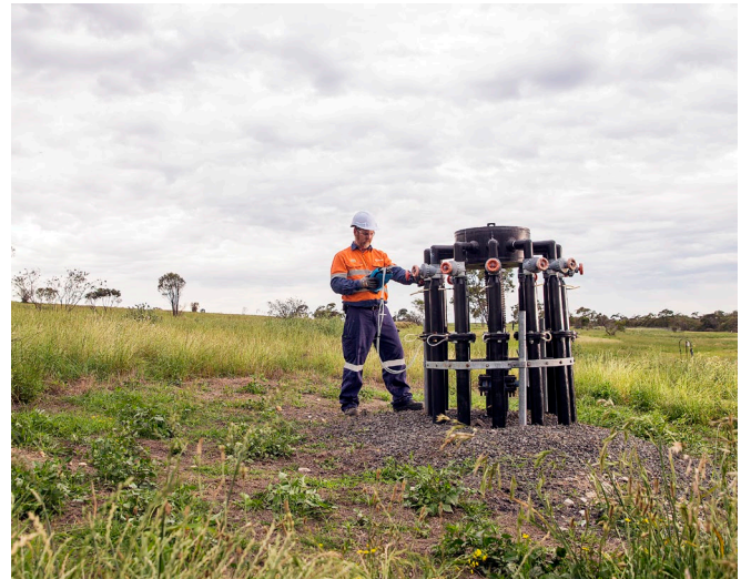
Lucas Heights landfill gas collection station
