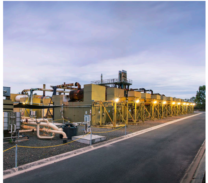
Lucas Heights Power Station
