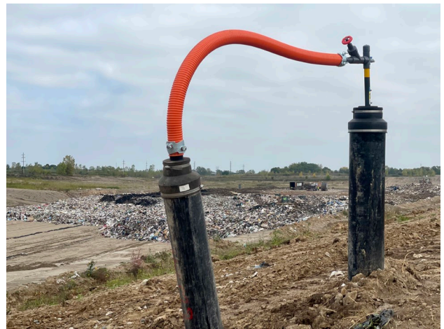
RNG will be created from waste gases from Granger Waste Services' Wood Street Landfill
