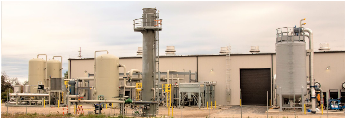
EDL's Wood Road RNG Facility
