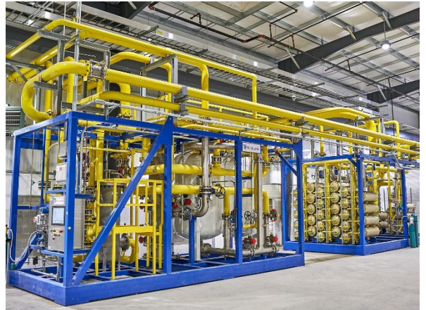
Air Liquide carbon dioxide removal system
