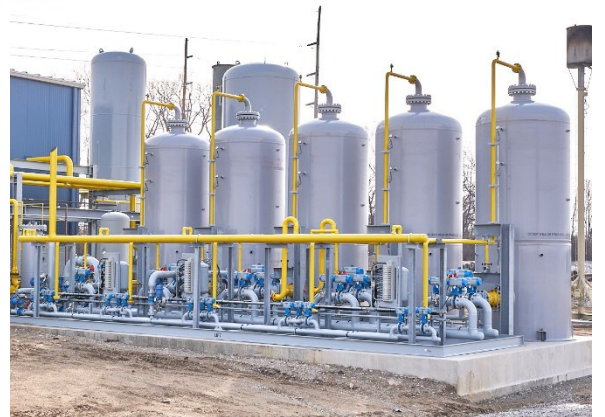
Guild Associates nitrogen removal system
