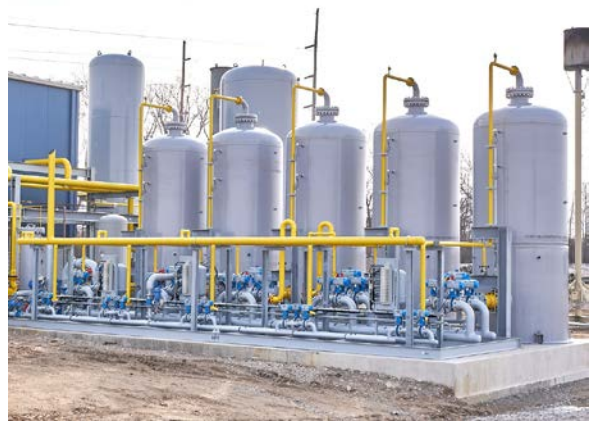
Guild Associates nitrogen removal system
