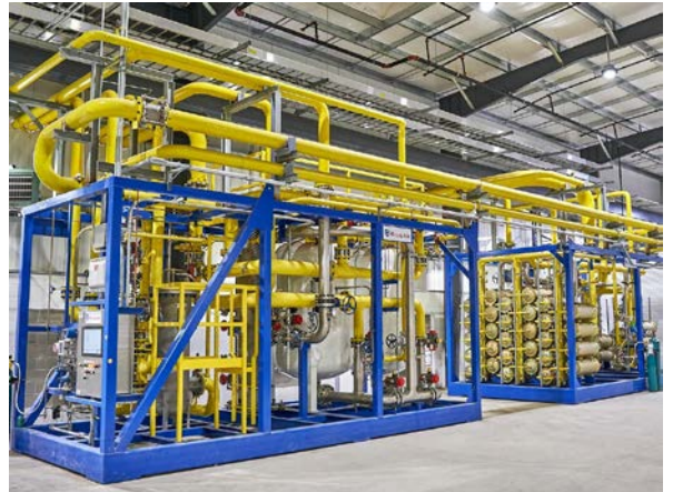
Air Liquide carbon dioxide removal system
