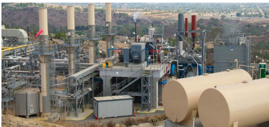
Brea LFG Plant
