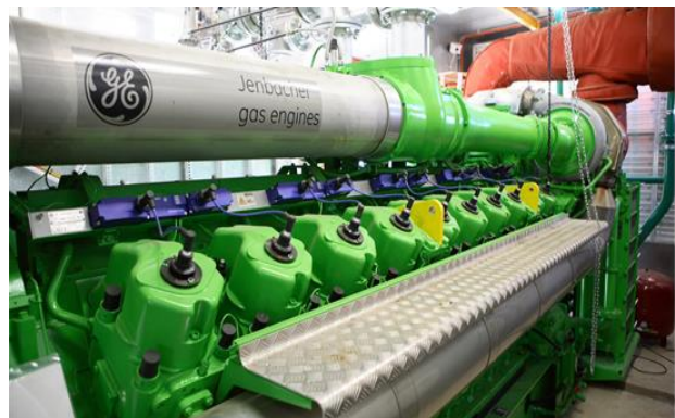
3MW power generation modules
