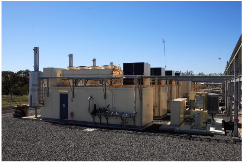
2MW power generation modules
