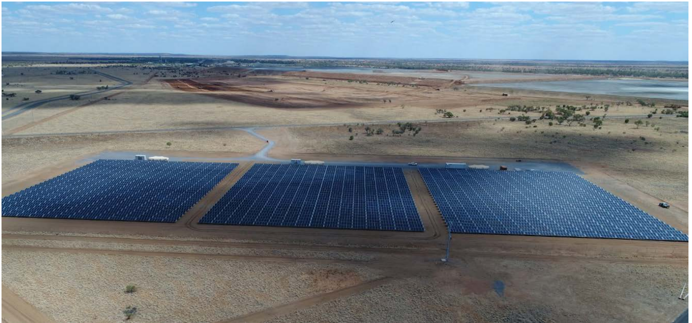
Solar PV facility at Cannington mine
