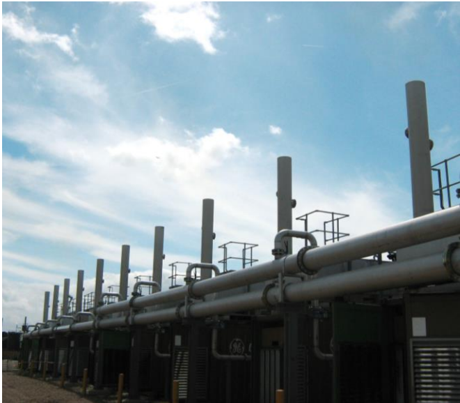
Pitsea Landfill Gas Power Station
