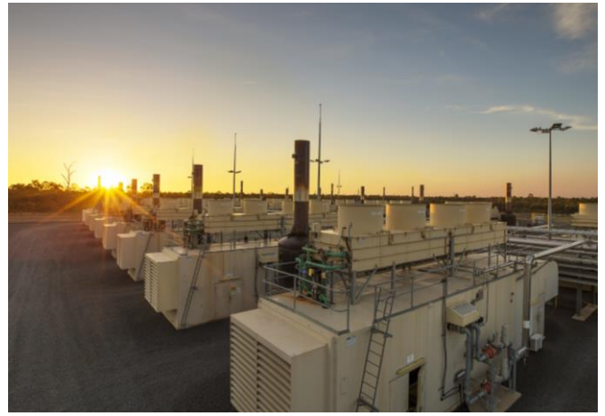
3MW power generation modules
