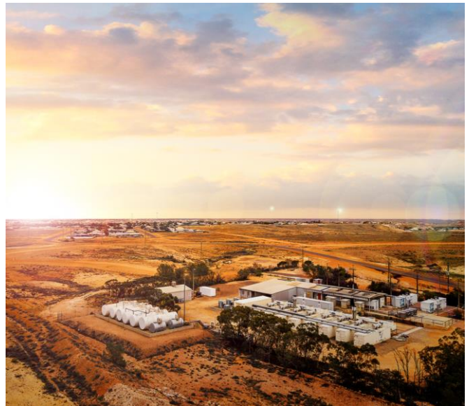
Coober Pedy Power Station
