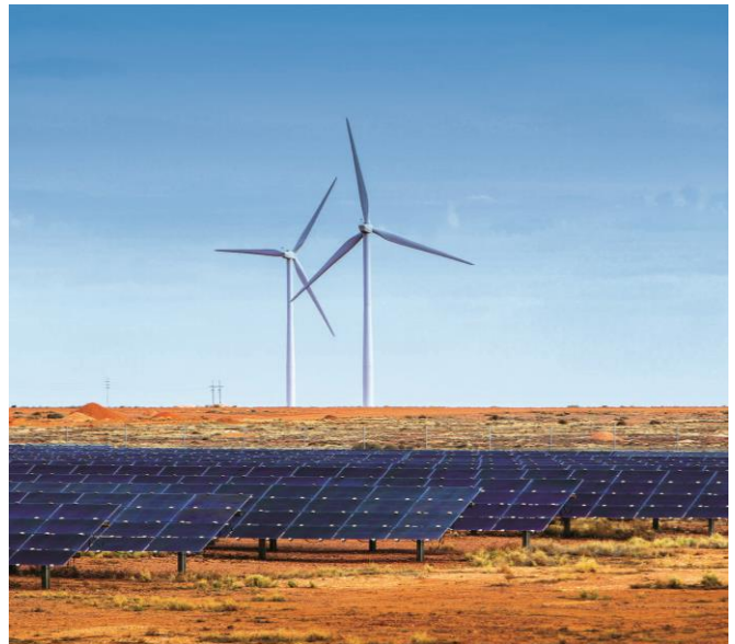
Coober Pedy solar and wind farm
