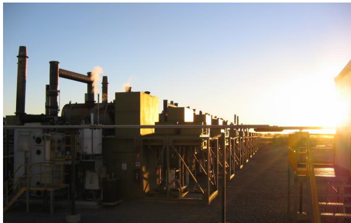
Power generation modules
